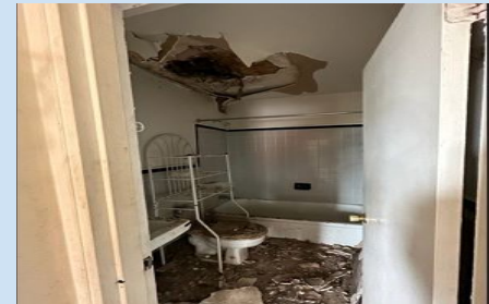
Collapsed ceiling in a bathroom of Averno Unit
